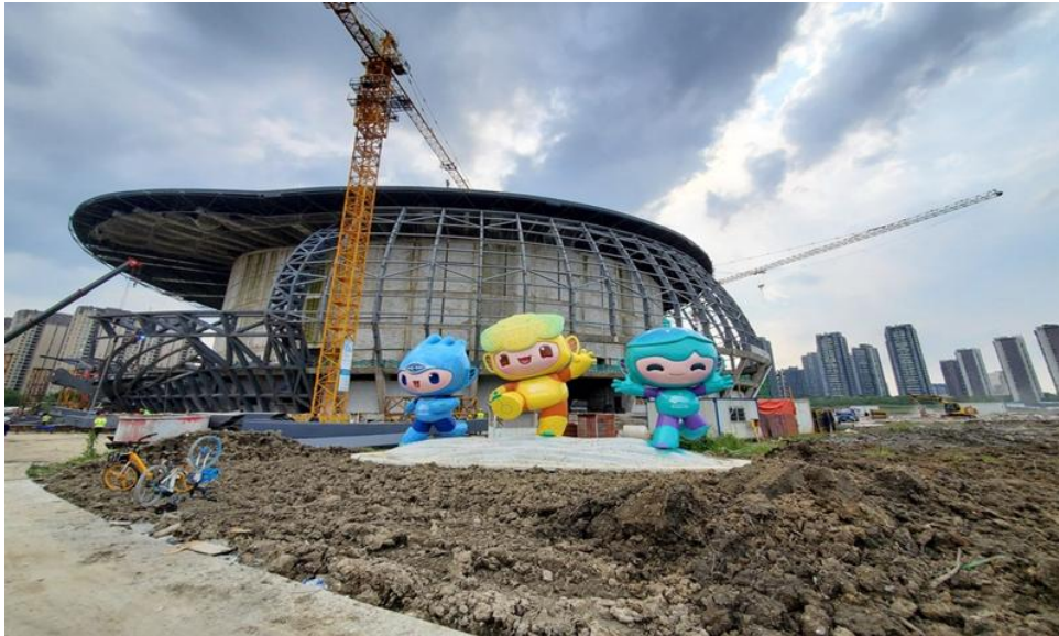
Construction site of the Gongshu District Chengxi Sports Park Stadium and Gymnasium. (Photo: Xinhua)
