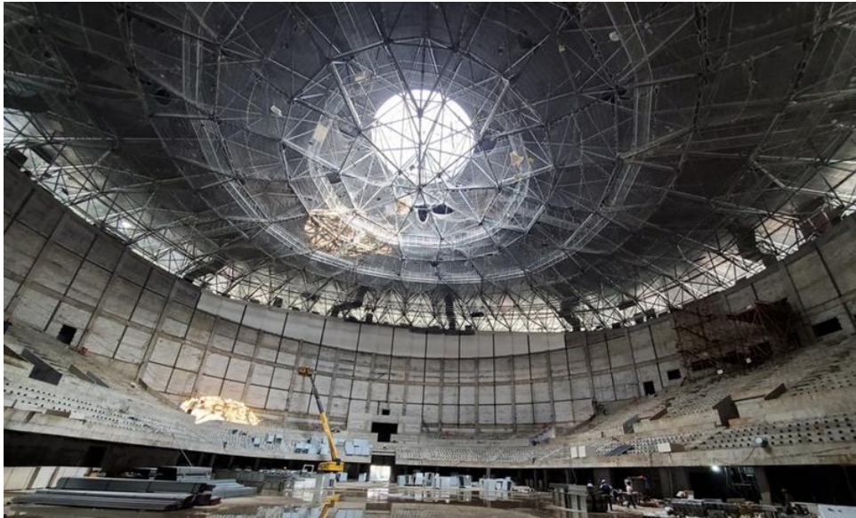
A view of the interior of the Sports Park under construction. (Photo: Xinhua)
